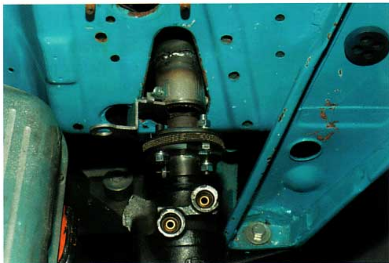
Photo #32: Install the coupler on the power steering box and make sure there is no interference with the bottom of the shift tube or shift lever. Readjusting of the lower mast jacket clamp left to right may be necessary.
